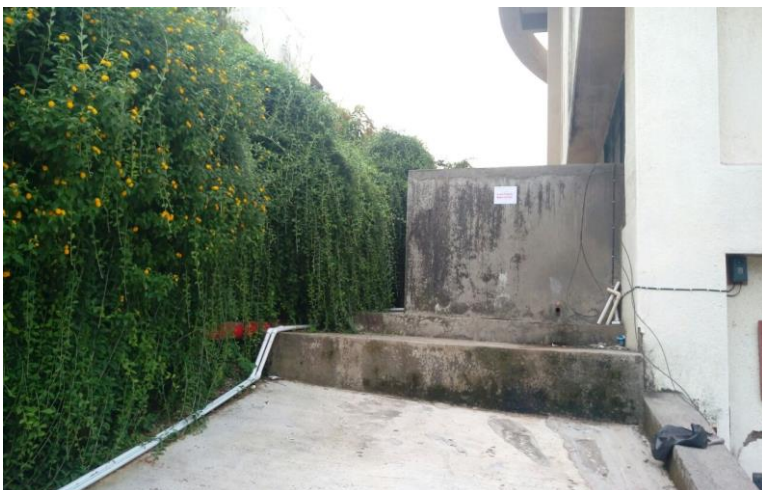
Rainwater harvesting tank
