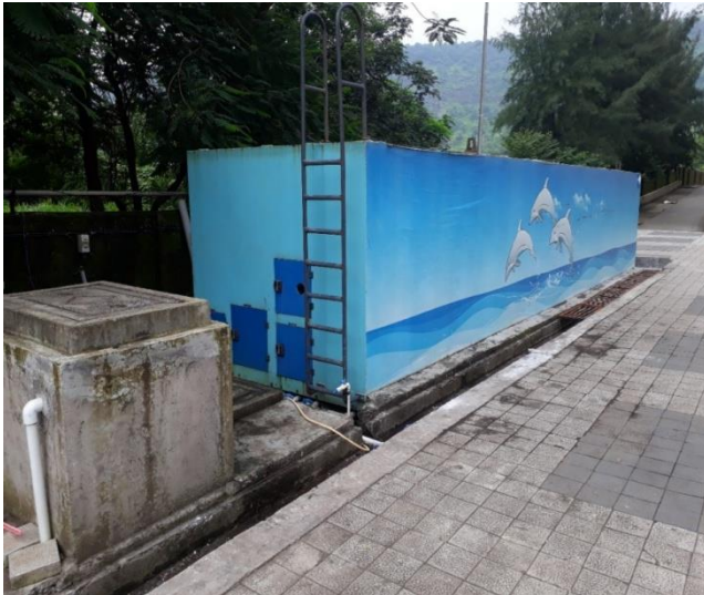
Sewage Treatment Plant of 1,00,000 lit per day filtration capacity
