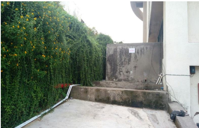
Rainwater harvesting tank
